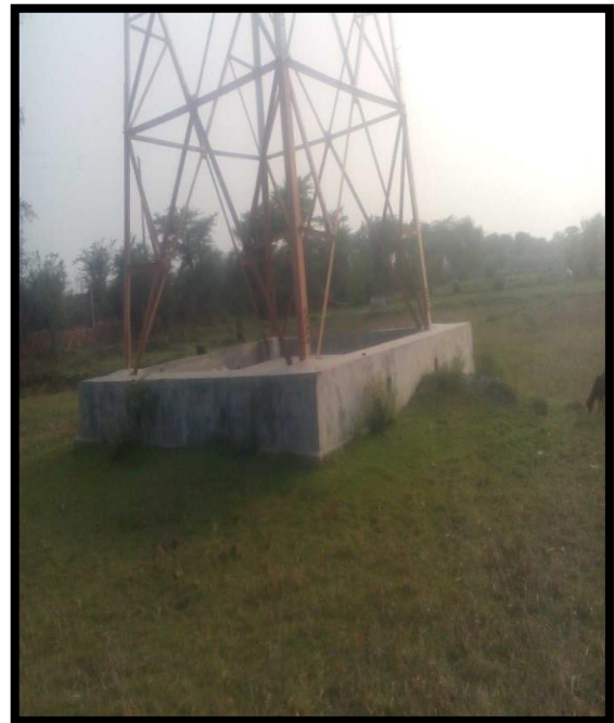
RIGHT RIVER BANK HIGH TENSION LINE AT CHAINAGE 49.5
