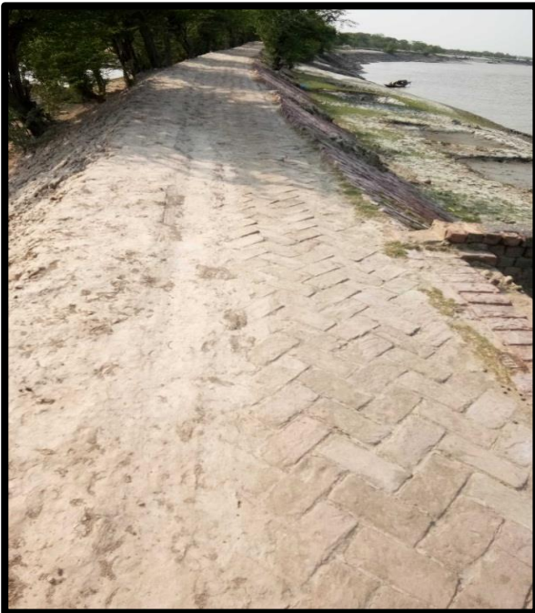
ROAD AT CHAINAGE 45.6, LEFT BANK
