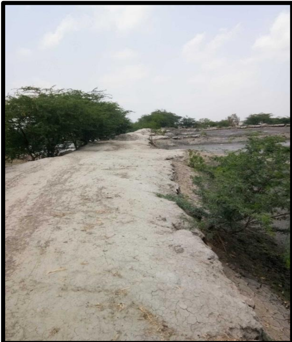
CHAINAGE 42.6, LEFT BANK
