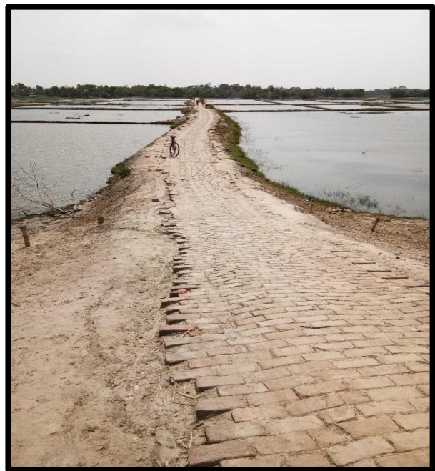
ROAD AT CHAINAGE 43.9, LEFT BANK
