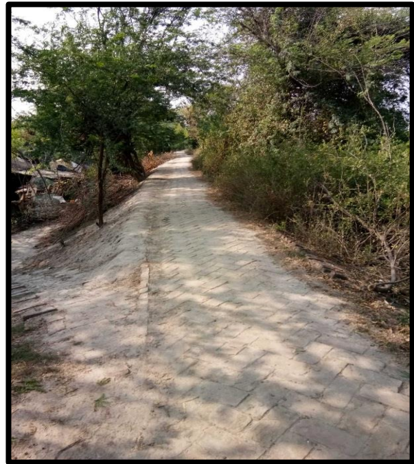
ROAD AT CHAINAGE 45.3, LEFT BANK
