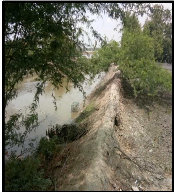
CHAINAGE 43.1, LEFT BANK
