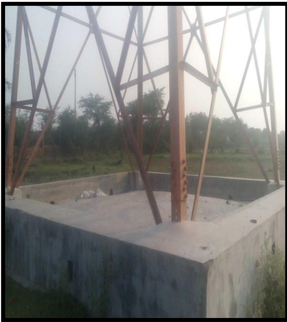
RIGHT RIVER BANK HIGH TENSION LINE AT CHAINAGE 49.5
