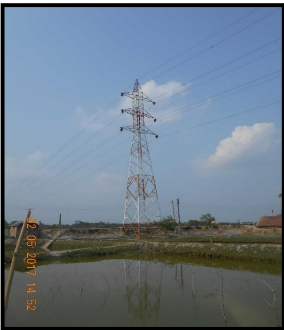
RIGHT RIVER BANK HIGH TENSION AT CHAINAGE 49.6
