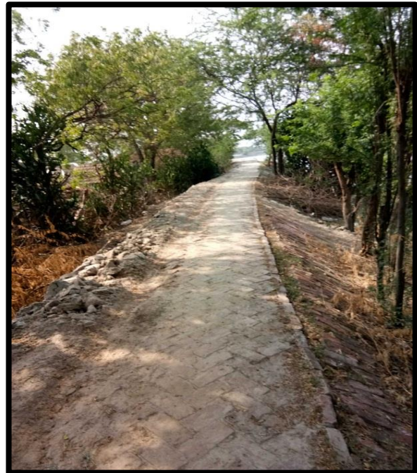
ROAD AT CHAINAGE 45.2, LEFT BANK
