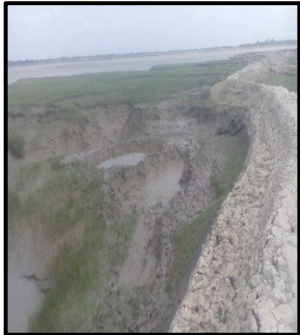
RIVER BANK AT CHAINAGE 24
