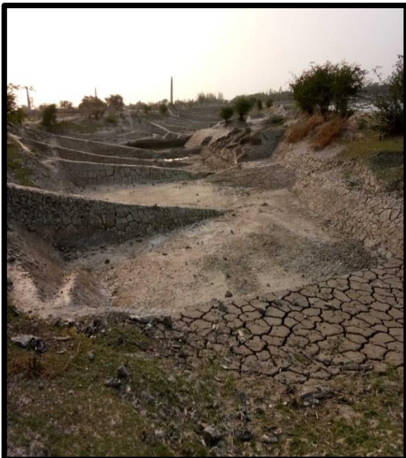
CHAINAGE 47.5, LEFT BANK
