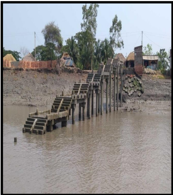
DAMAGED JETTY AT CHAINAGE 29.5, RIGHT BANK
