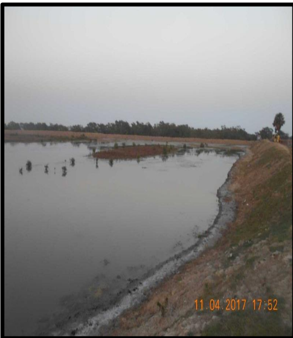
Pond at Left Bank Chainage 21.6
