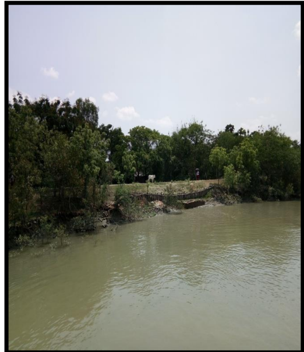
Damaged Right River Bank Protection at Chainage 43
