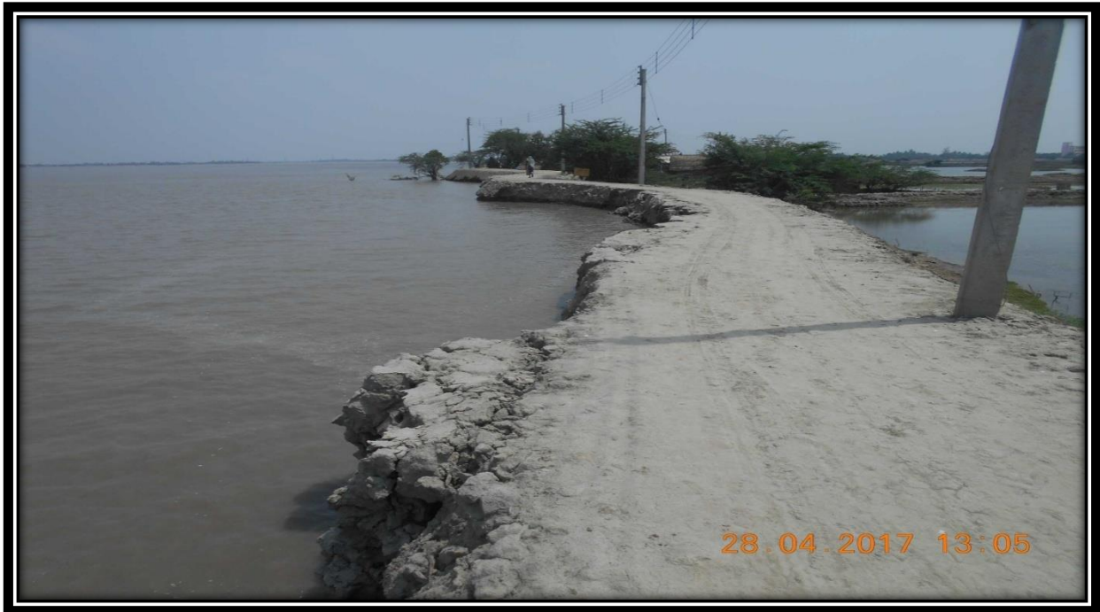
Soil Erosion at Chainage 9.0
