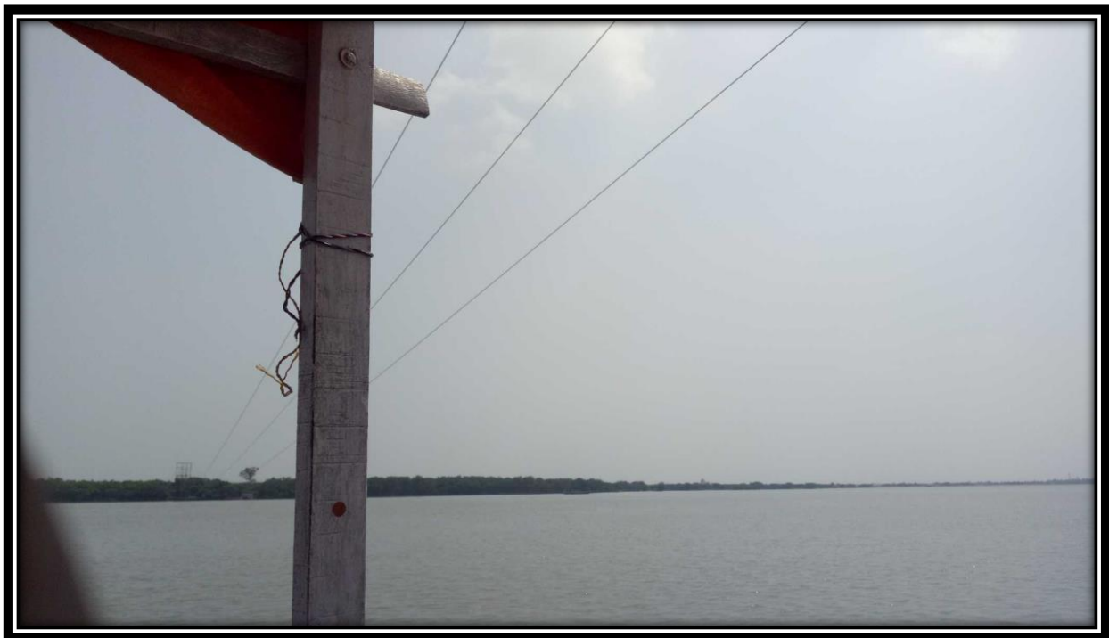
Electric Line Crossing at Chainage 15.0
