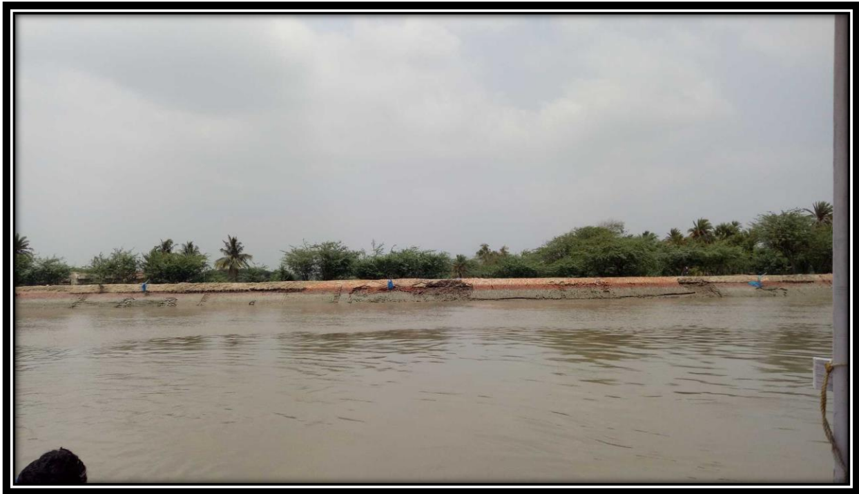
Damaged Protected Bank at 7.2
