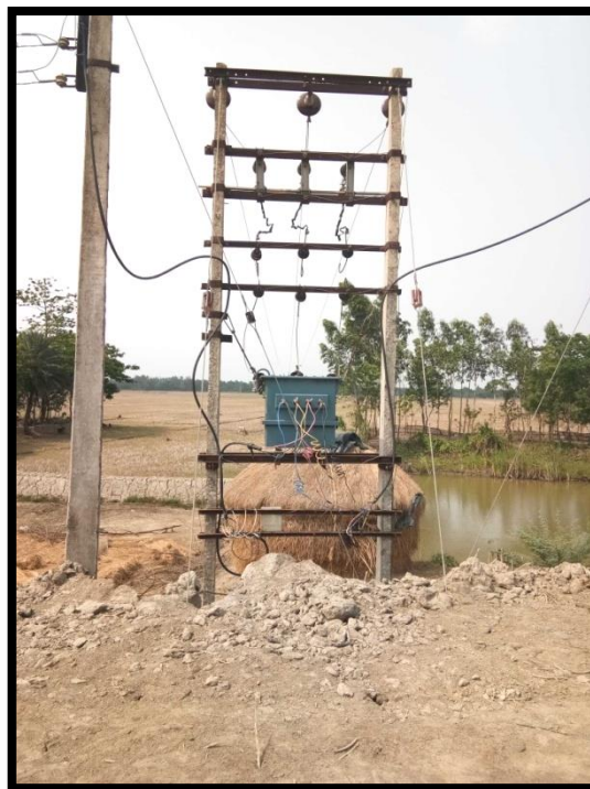
Transformer at Chainage 5.8
