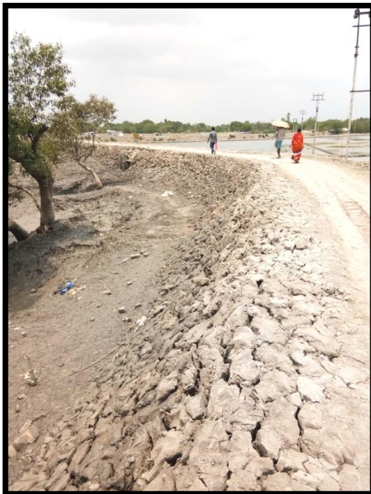
Road on right bank of river at chainage 4.4
