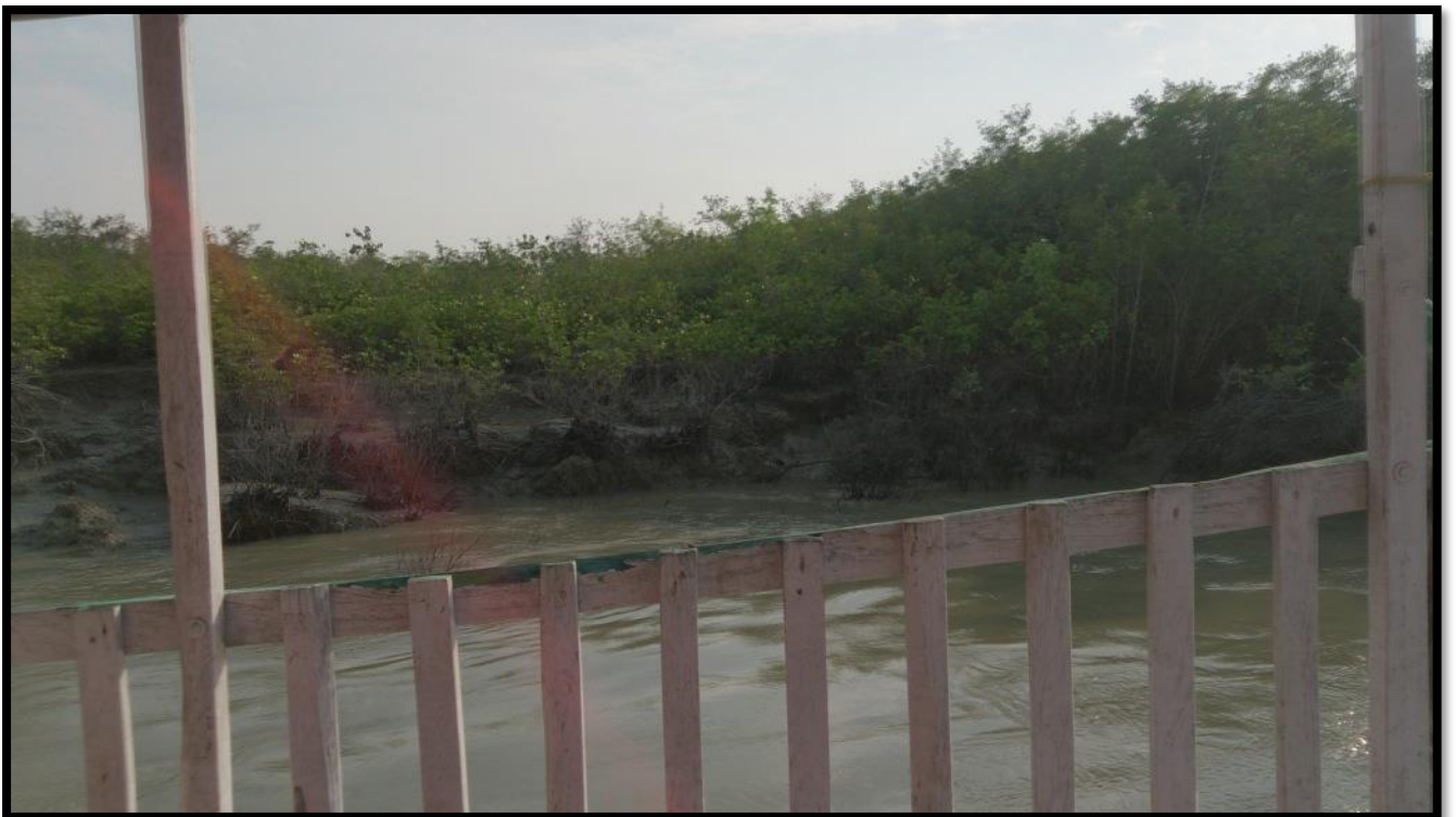
Unprotected Right Bank at CHAINAGE 5.6
