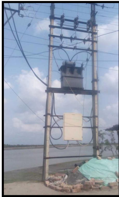
Transformer at Chainage 7.8
