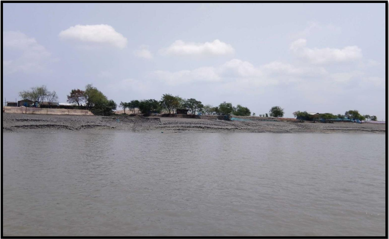
Unprotected Bank at Chainage 4.8
