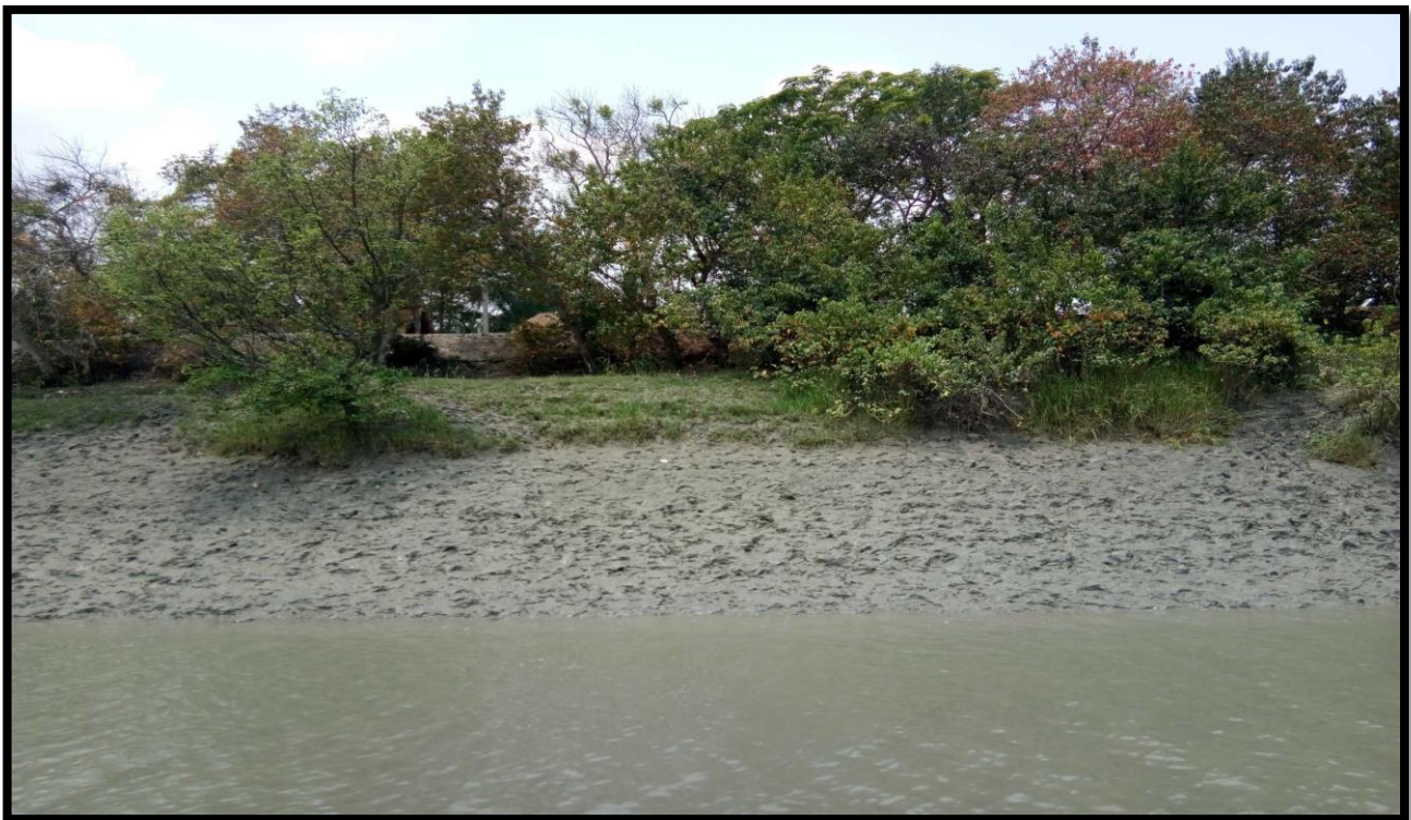
Unprotected Left Bank at CHAINAGE 6.5
