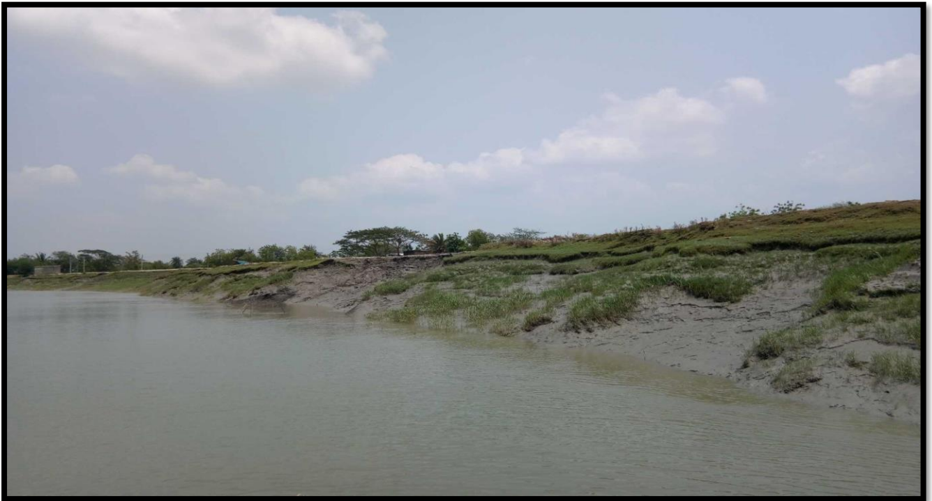
Unprotected Right Bank at CHAINAGE 14.5
