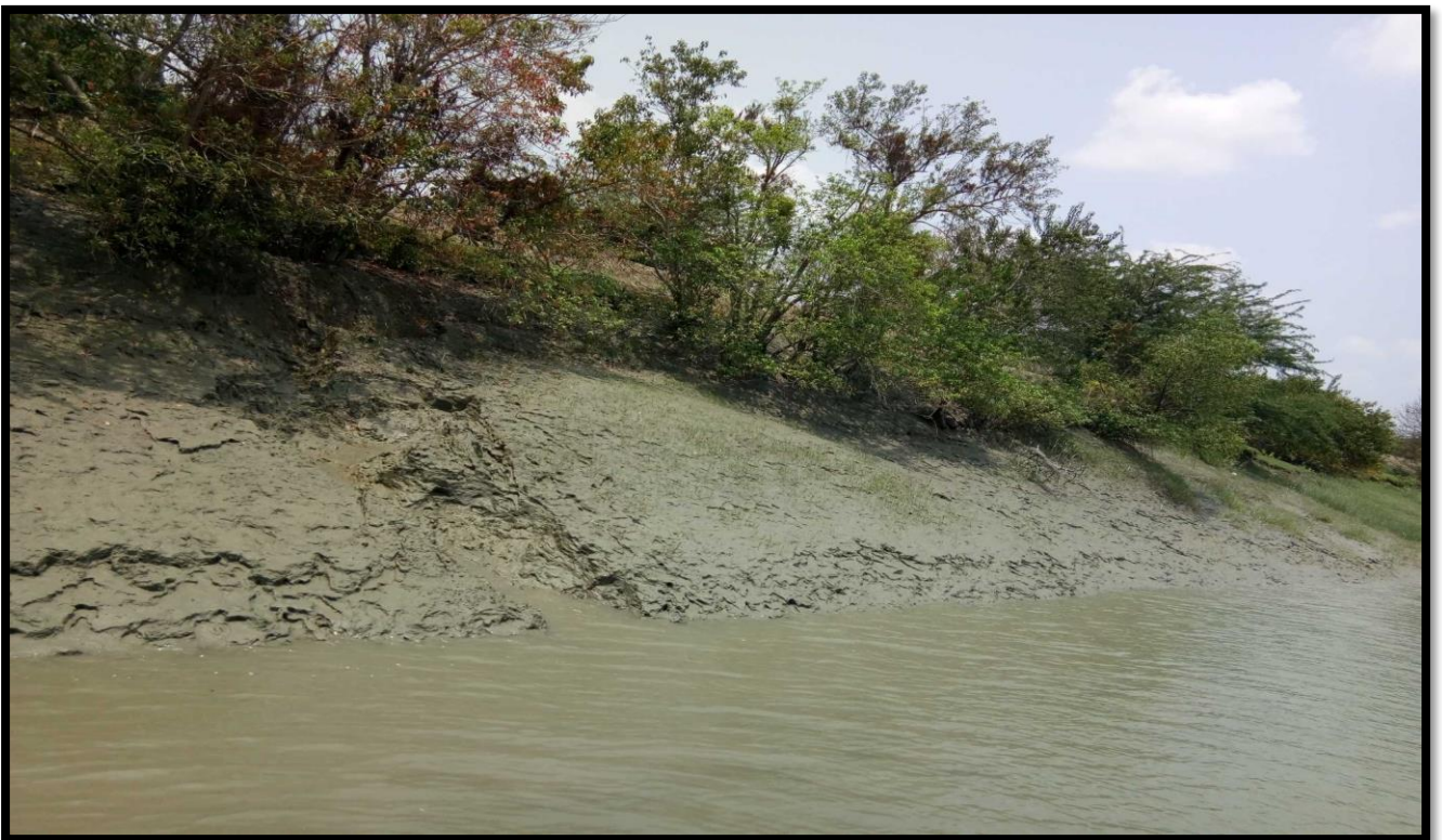
Unprotected Left Bank at CHAINAGE 12.0
