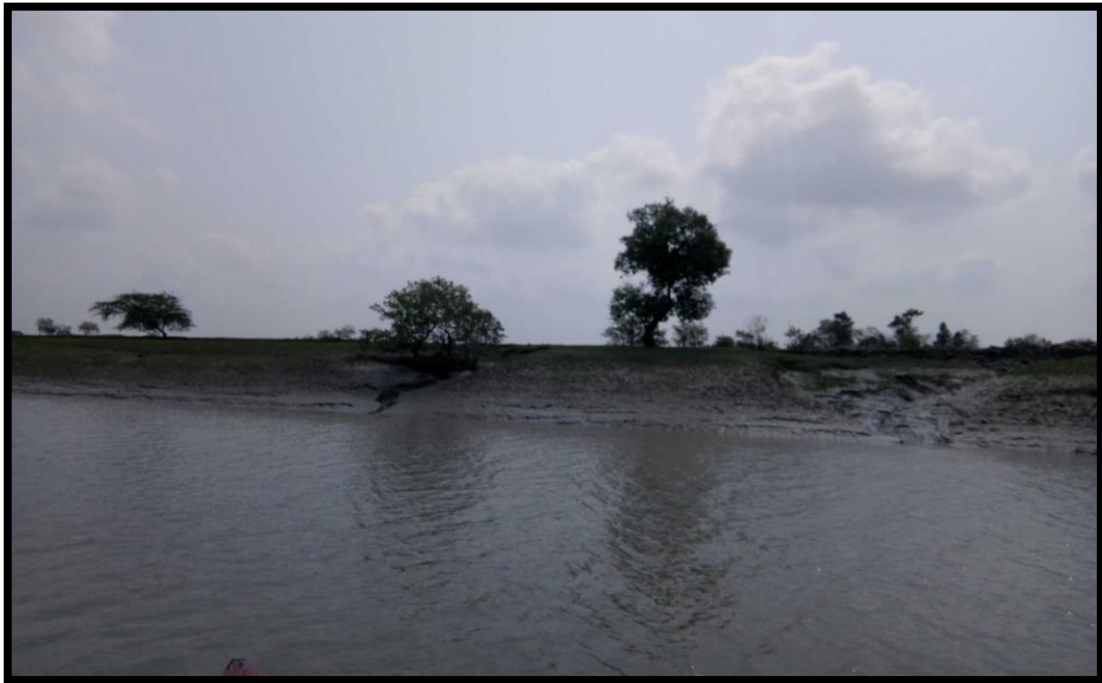
Unprotected Right Bank at CHAINAGE 2.0
