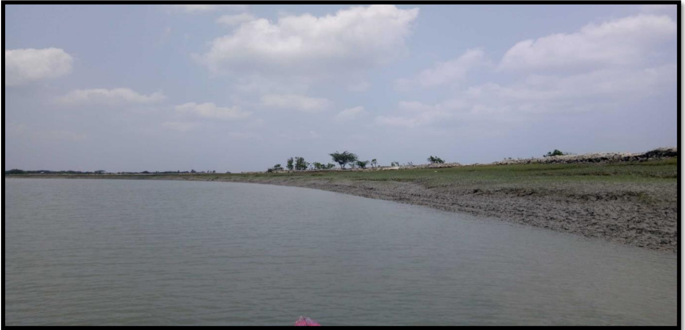
Unprotected Right Bank at CHAINAGE 11.0
