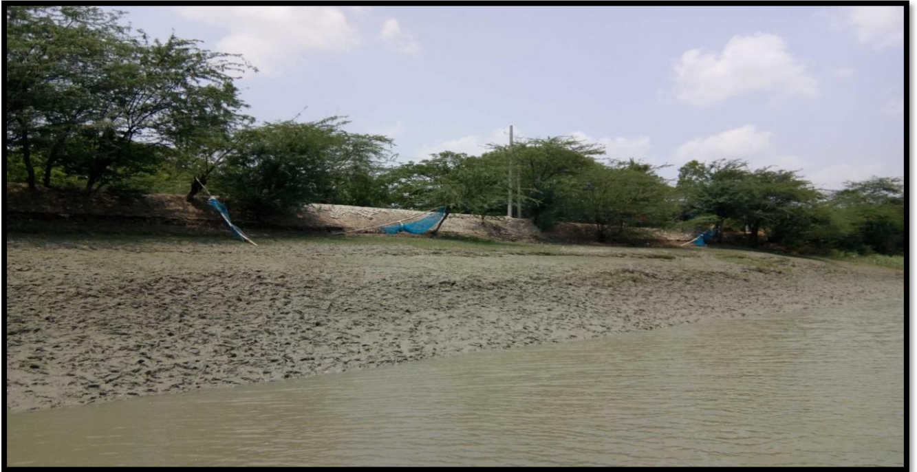
Unprotected Left Bank at CHAINAGE 12.5
