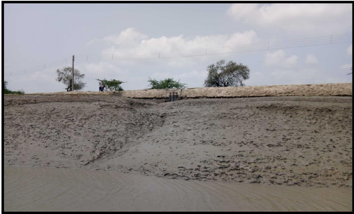
Unprotected Left Bank at CHAINAGE 4.5
