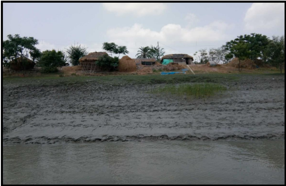
Unprotected Left Bank at CHAINAGE 3.5
