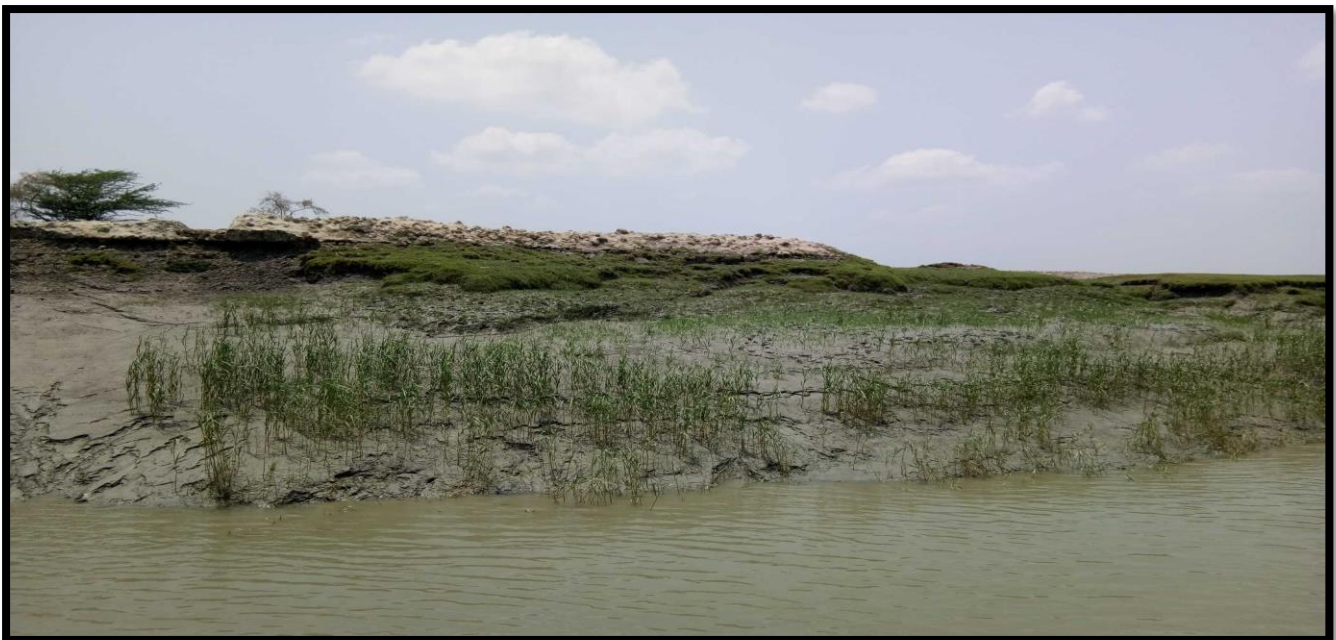
Unprotected Left Bank at CHAINAGE 15.0
