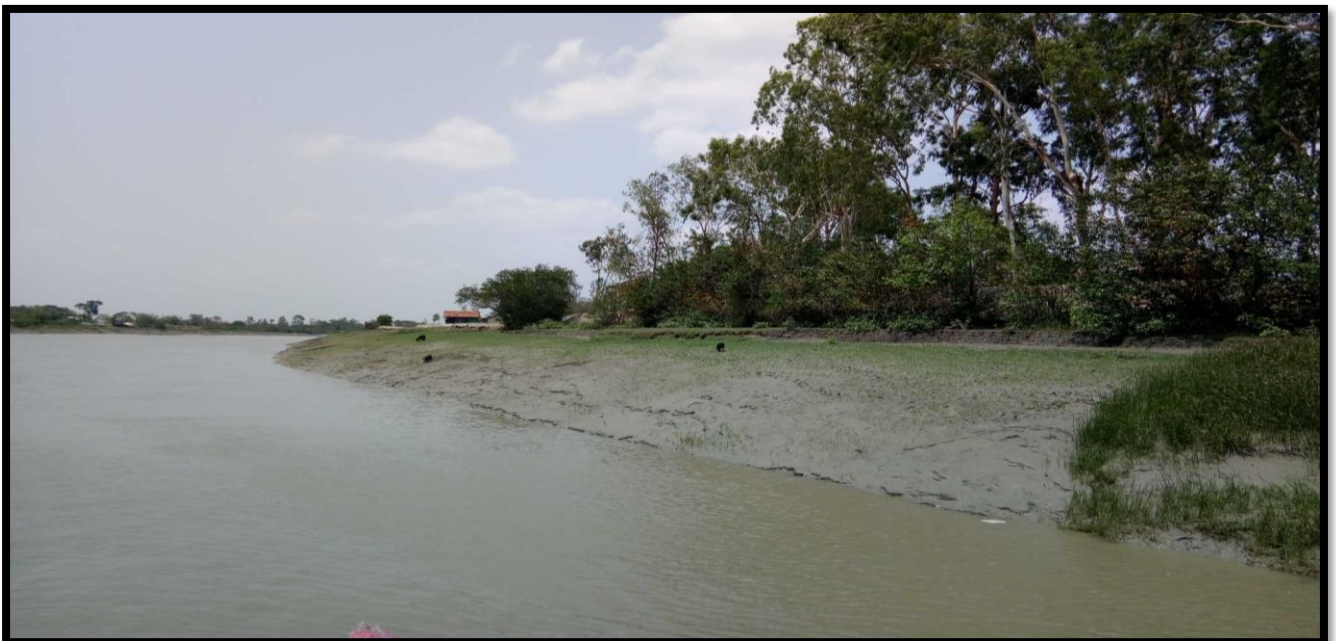
Unprotected Right Bank at CHAINAGE 17.0
