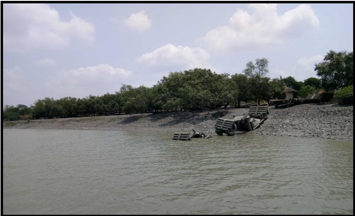
Broken Ferry Jetty at 4.0 CHAINAGE on Right Bank
