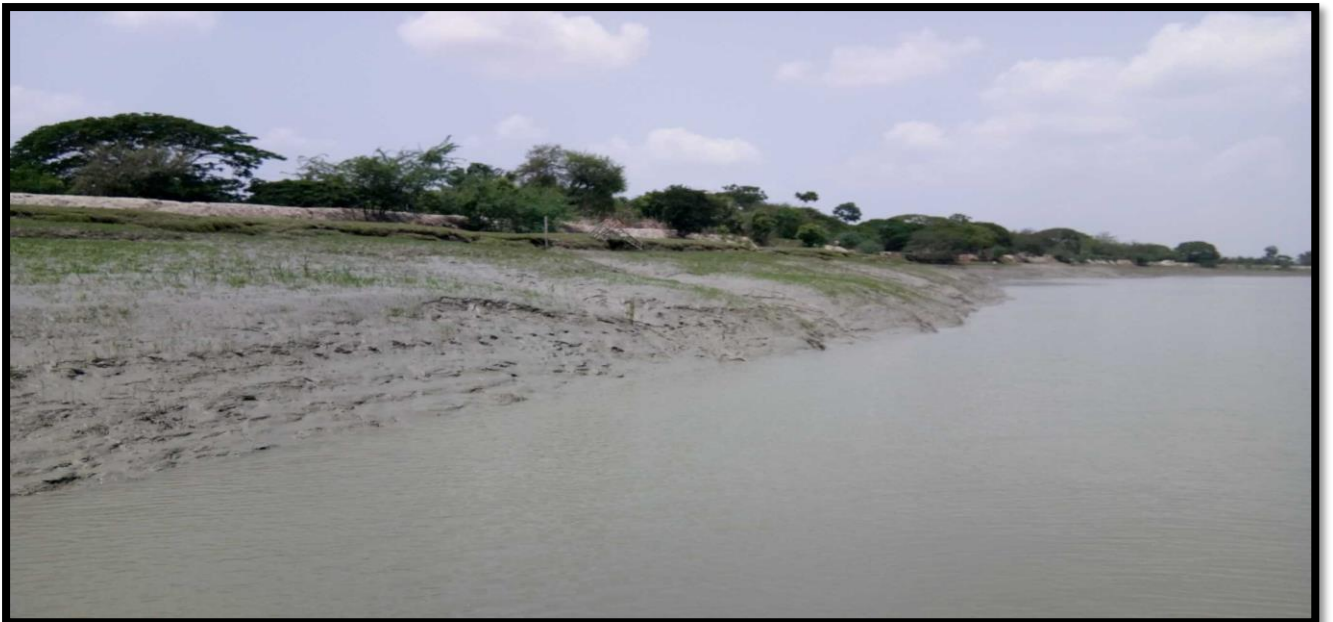
Unprotected Left Bank at CHAINAGE 10
