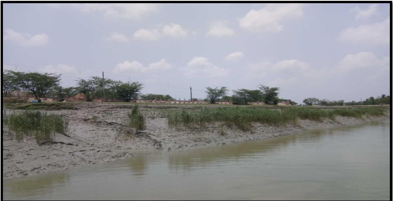
Unprotected Left Bank at CHAINAGE 11.5
