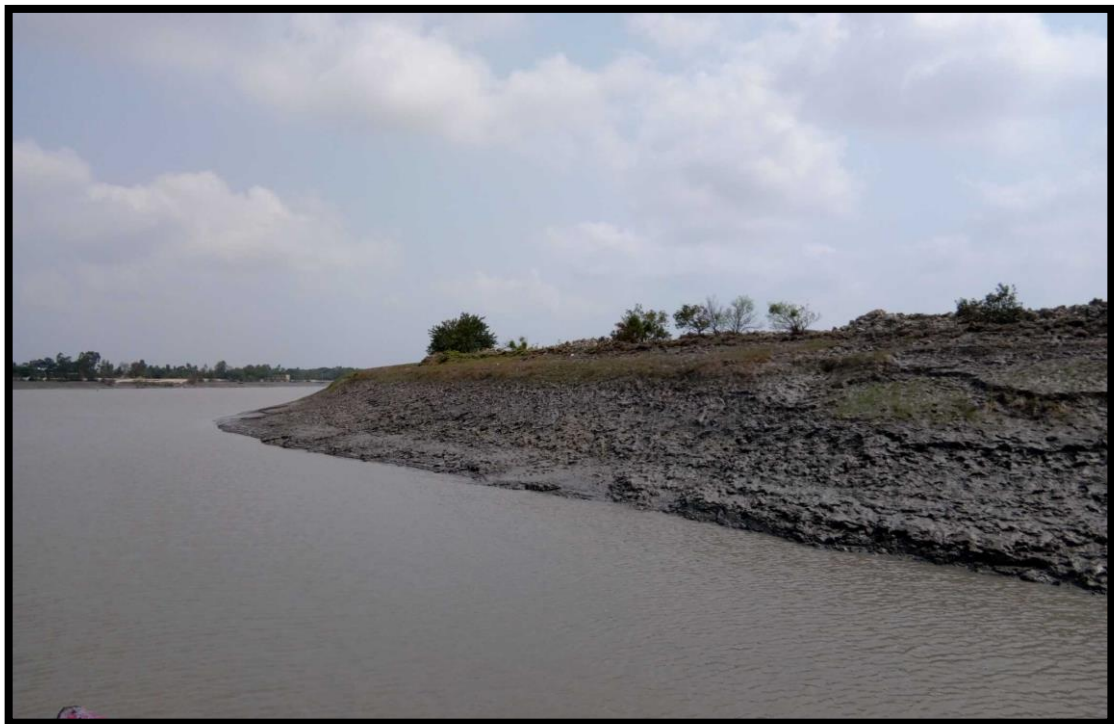
Unprotected Right Bank at CHAINAGE 1.5
