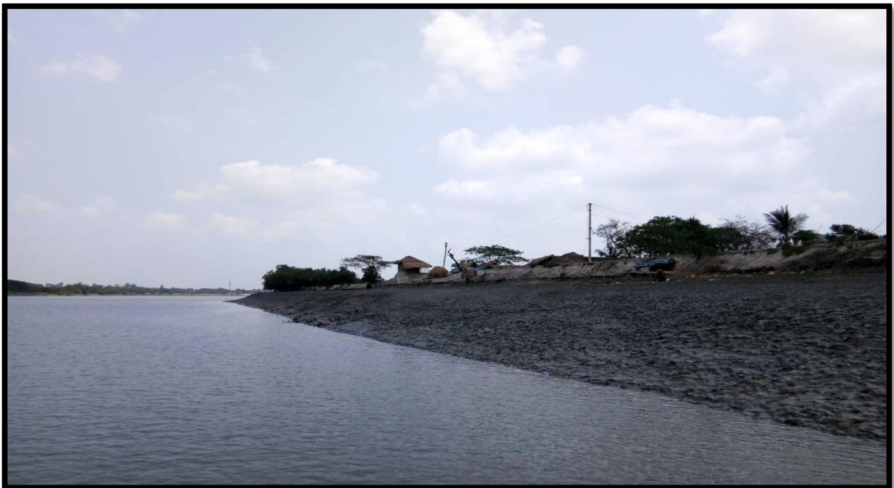
Unprotected Right Bank at CHAINAGE 6.5
