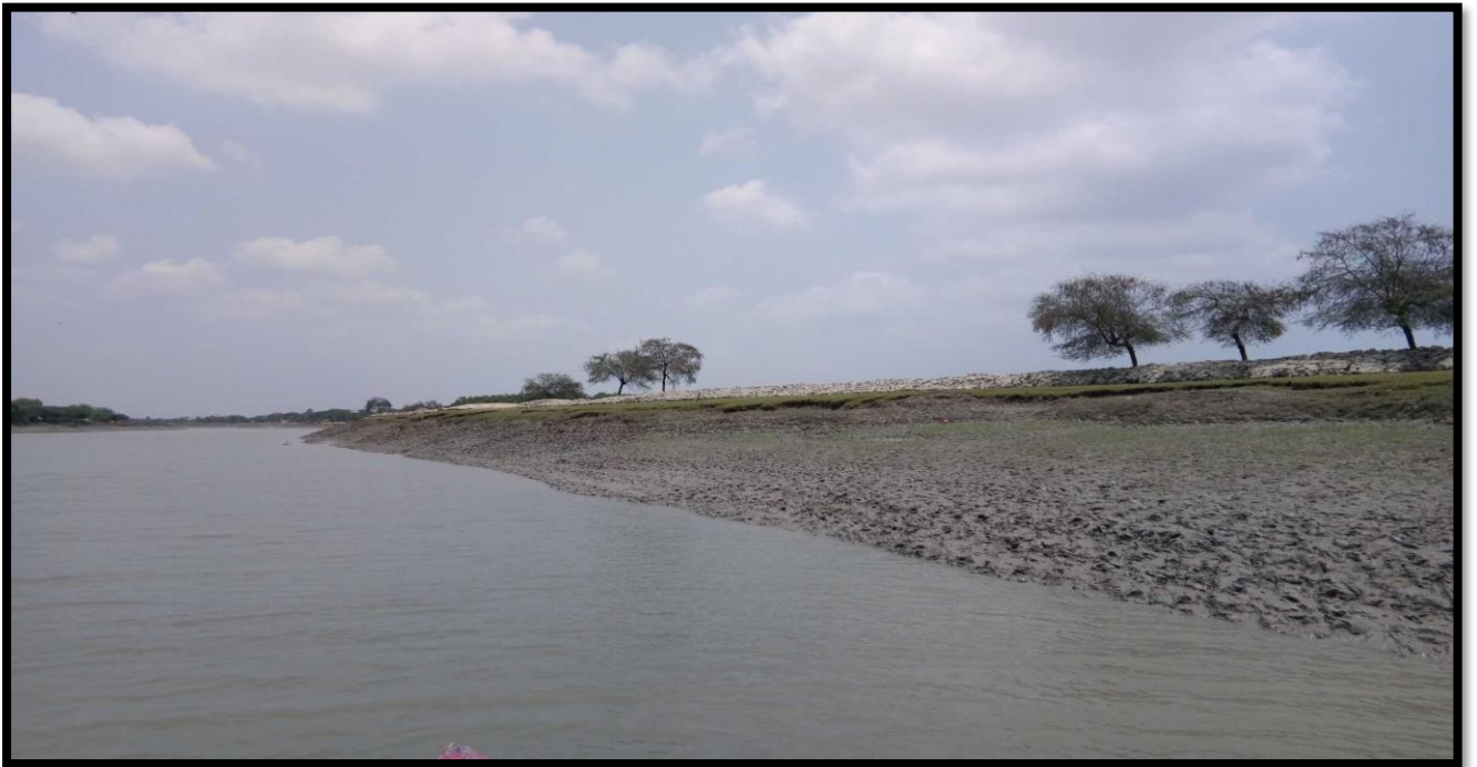
Unprotected Right Bank at CHAINAGE 9.5
