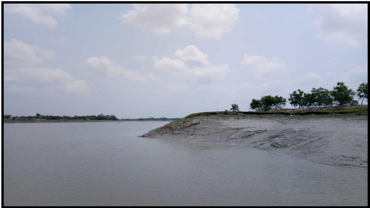
Unprotected Right Bank at CHAINAGE 5.0
