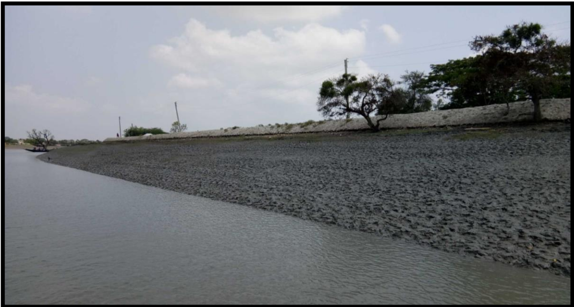
Unprotected Right Bank at CHAINAGE 3.5
