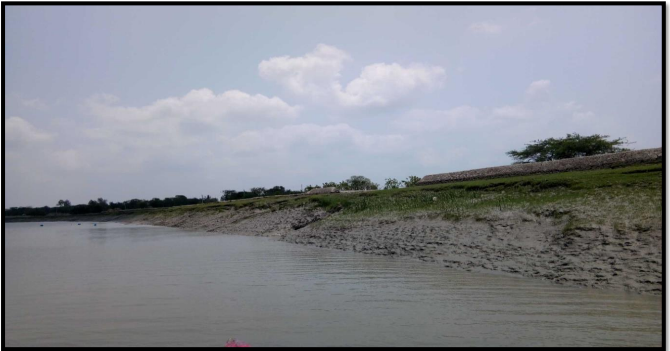
Unprotected Right Bank at CHAINAGE 9.0
