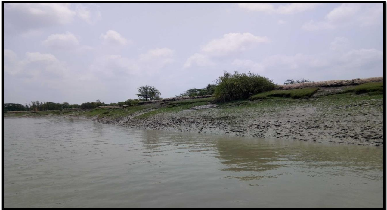
Unprotected Right Bank at CHAINAGE 5.5
