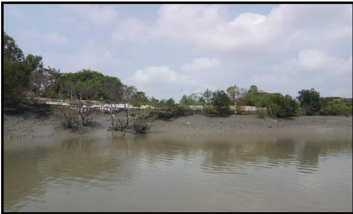
Unprotected Right Bank at CHAINAGE 1.0
