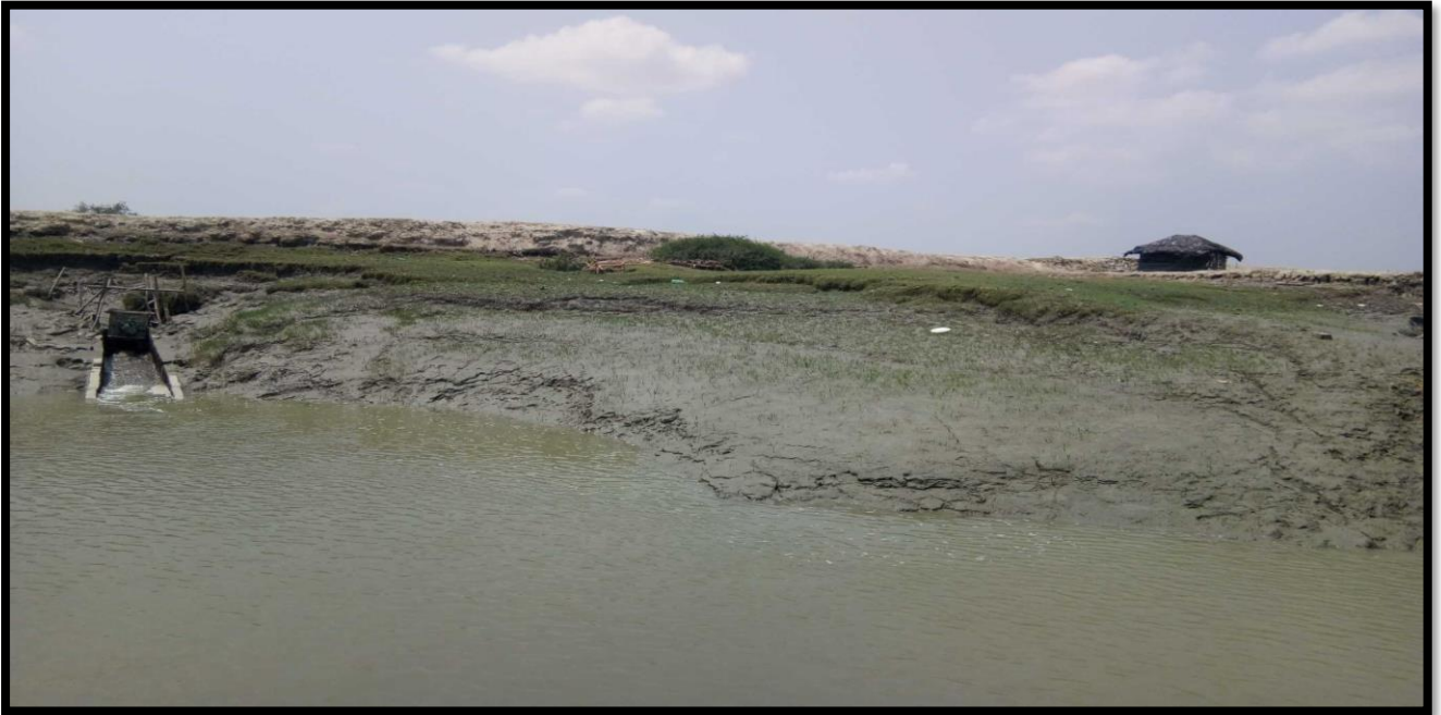
Unprotected Left Bank at CHAINAGE 20.0
