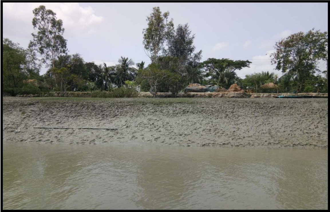
Unprotected Left Bank at CHAINAGE 3.0
