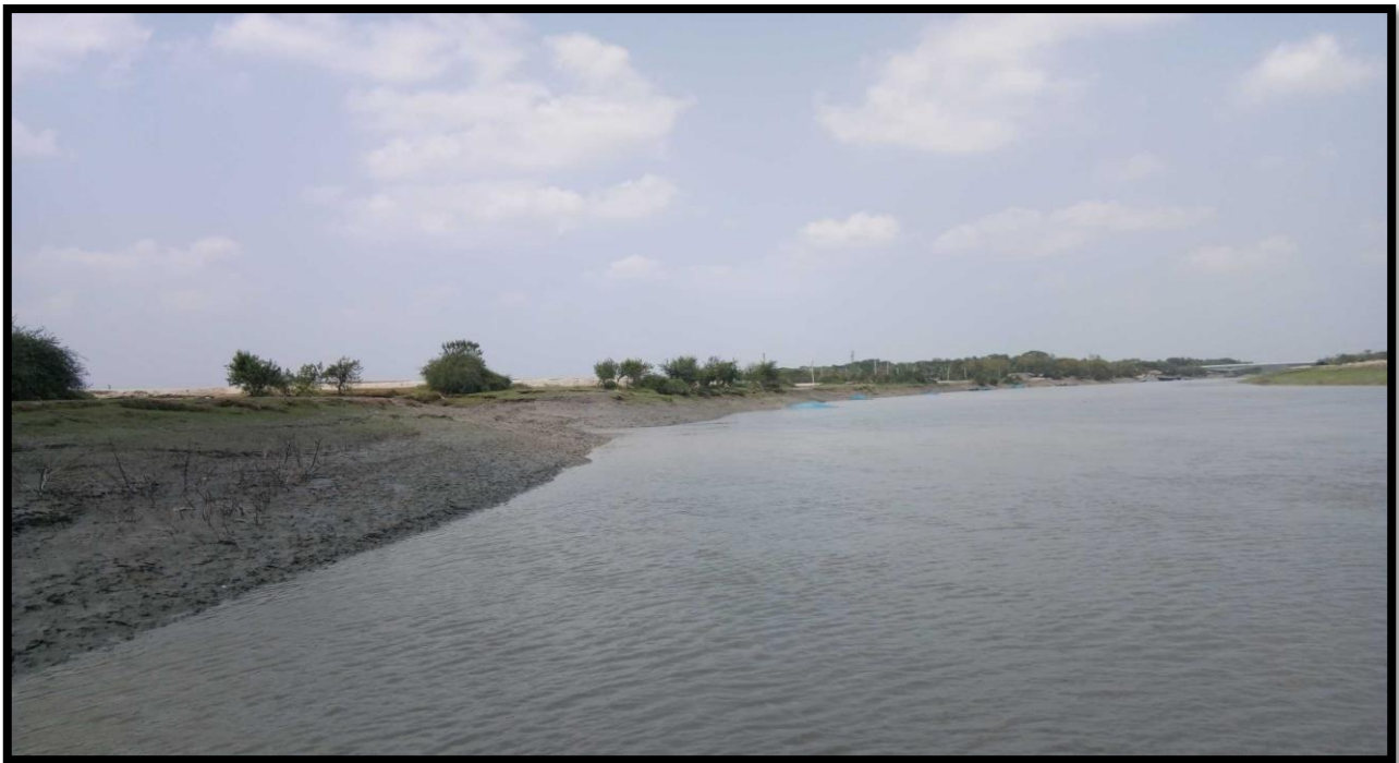
Unprotected Left Bank at CHAINAGE 21.5
