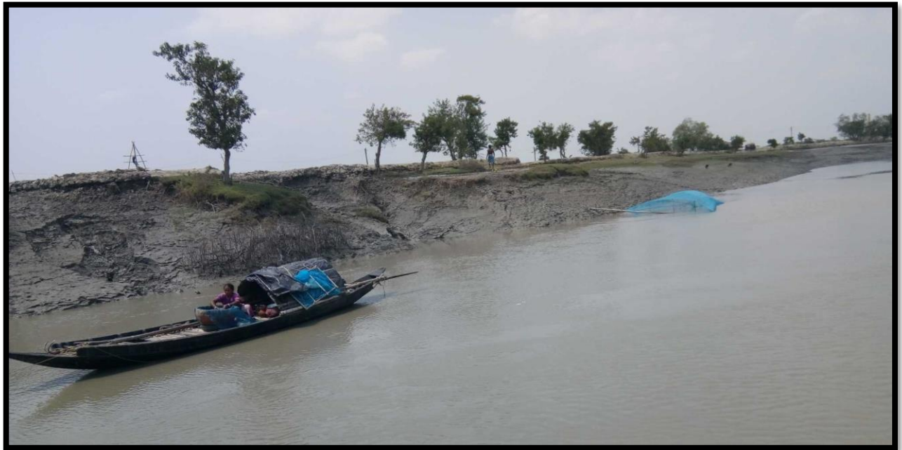
Fishing activity on unprotected Left Bank at CHAINAGE 20.5
