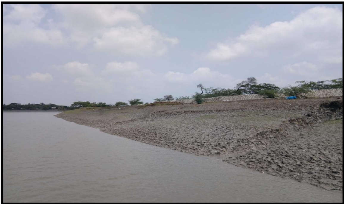
Unprotected Right Bank at CHAINAGE 4.5
