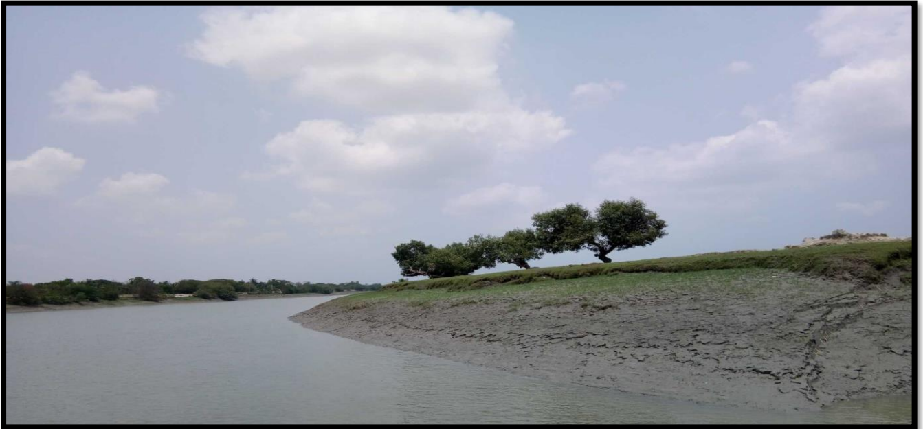
Unprotected Right Bank at CHAINAGE 12.0
