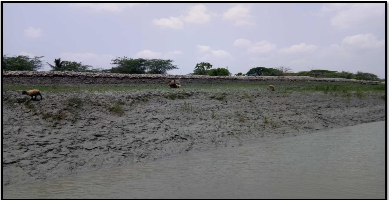
Unprotected Left Bank at CHAINAGE 11.0
