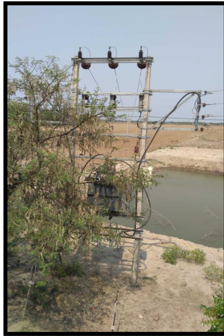
Transformer Pole at Chainage 10.3
