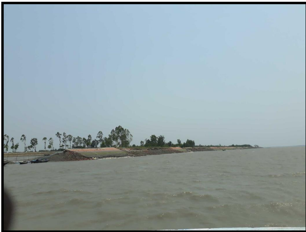
River Bank condition at Chainage 4.5
