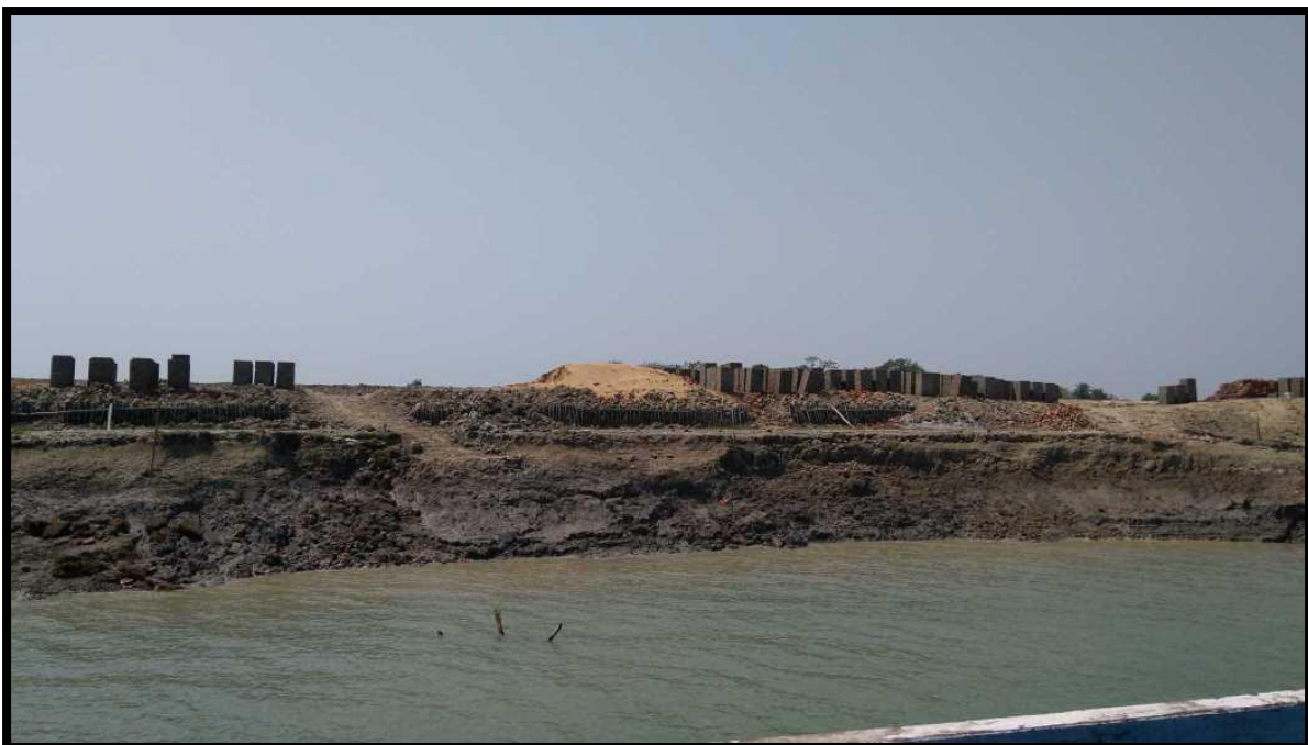
Soil Erosion at Chainage 19.5
