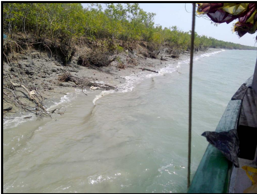
Unprotected River Bank at Chainage 12.5
