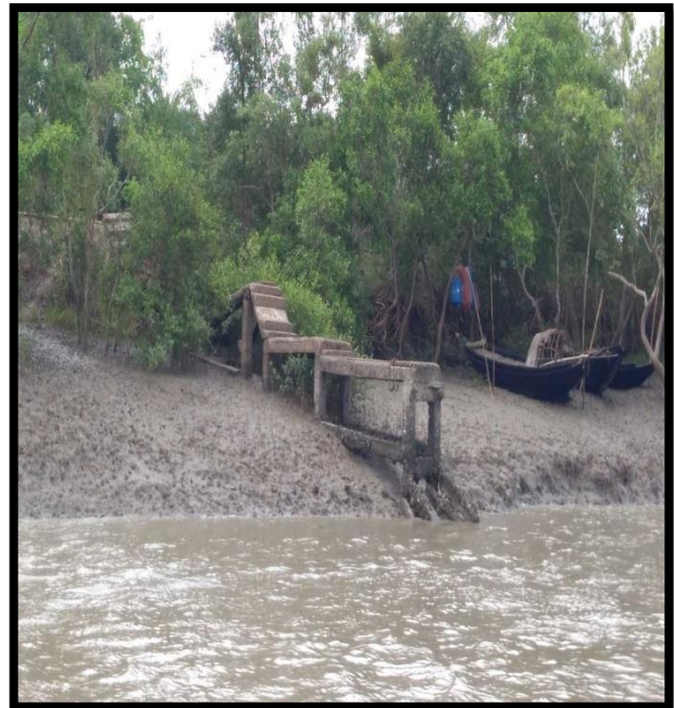
Right River Bank Broken Bhunesvar Jetty at Chainage 41.4
