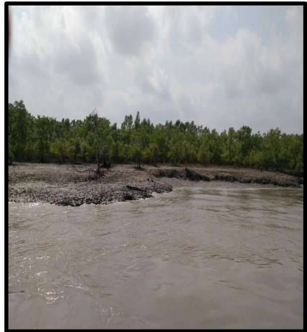
Soil Erosion Area at Left Bank Chainage 31.6
