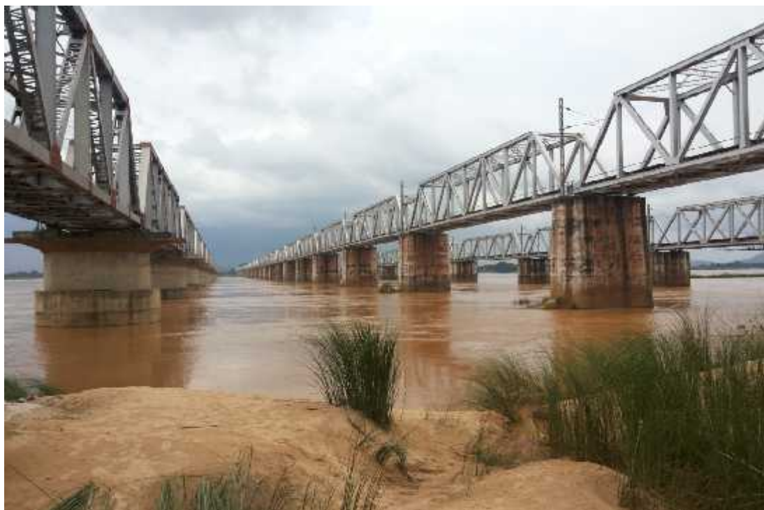
Figure No. 3-1 A view of Railway Bridge at Pankapal during August 2014 floods
