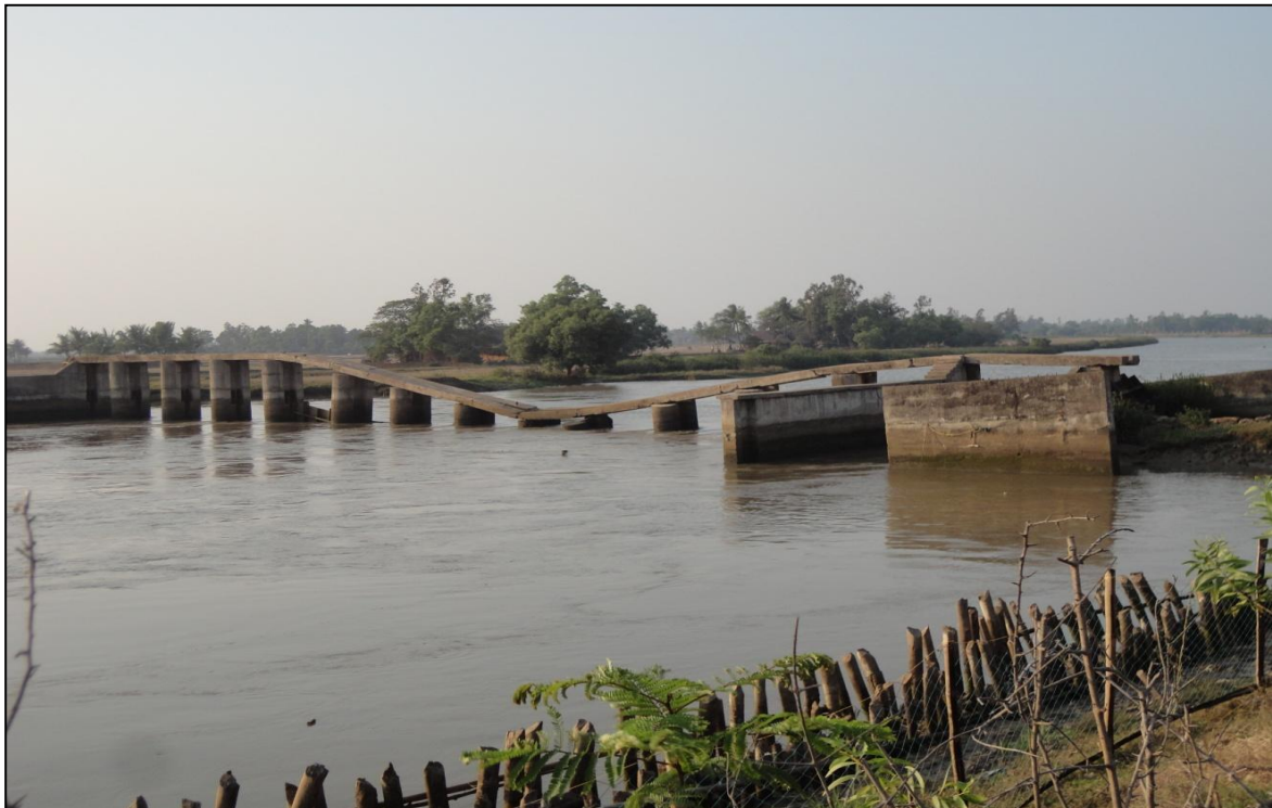
Photo 36 : Damaged Bridge on Nuna Creek
