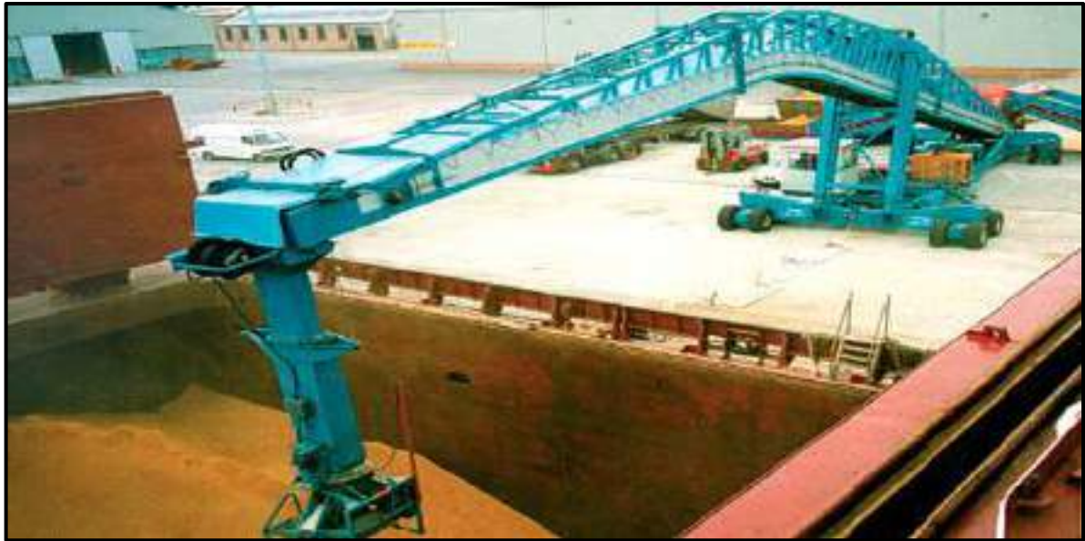
Figure 10.1: Typical Mobile Barge Loader
