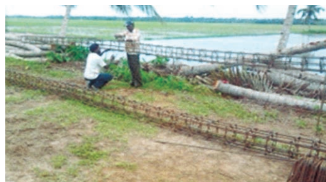
A view on the steel fabrication work for piles in Kuttanad area by M/s Yojaka (India) Ltd.
